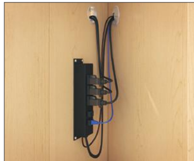
Module interior - Power/Voice/Data connections and access
